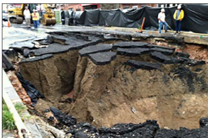
Figure 3. Monument Street sinkhole that occurred on August 26, 2012.
